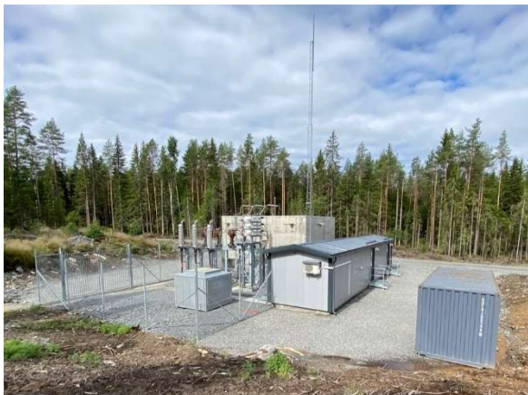
Figur 15. Transformatorstation i Marker Vindpark, Norge.
