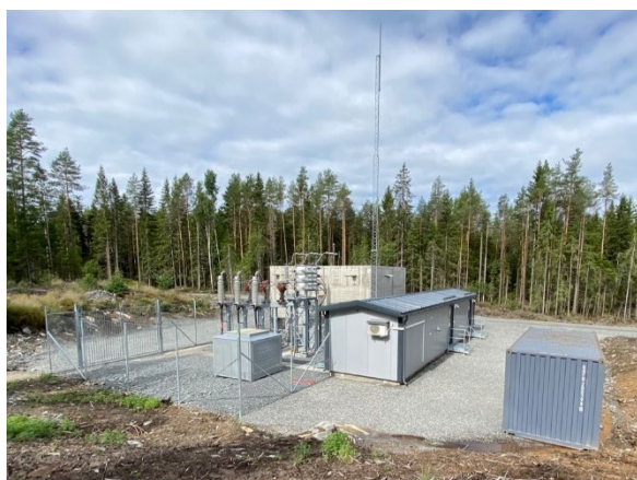
Figur 12 Transformatorstation i Marker Vindpark, Norge
