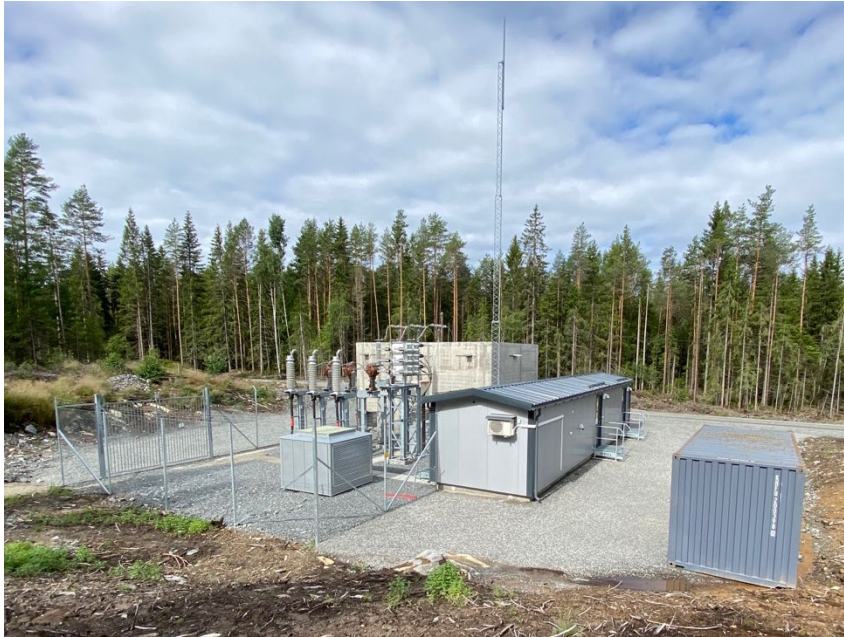
Figur 12 Transformatorstation i Marker Vindpark, Norge
